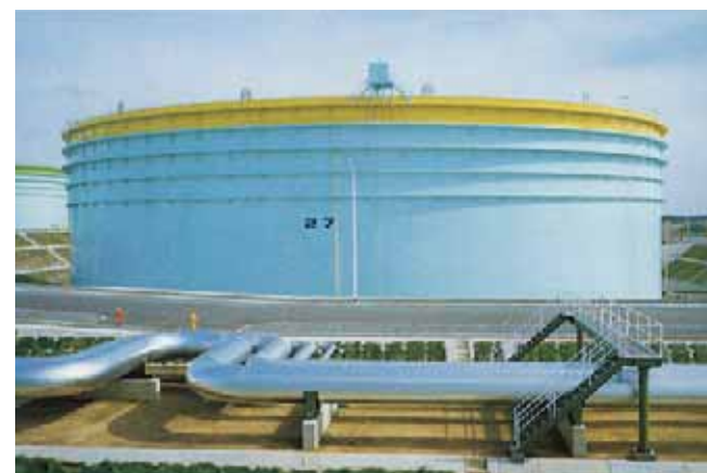
Crude oil storage tanks
